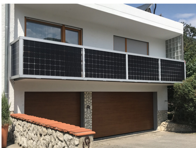
PV Power Wall Balcony (1.6 kWp)
