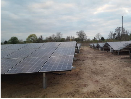
3150 kWp in Coburg, Germany
