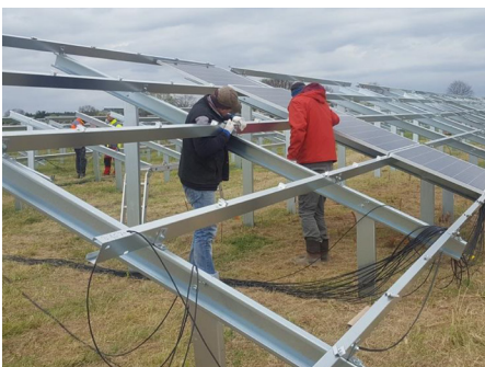
750 kWp in Pakendorf, Germany
